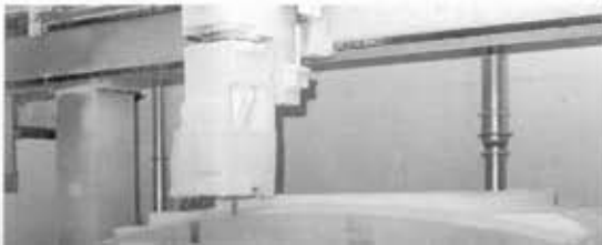
3.16a–c. The double-curved acrylic glass panels for Bernhard Franken's "Bubble" BMW pavilion (1999) were produced using CNC-milled molds.
